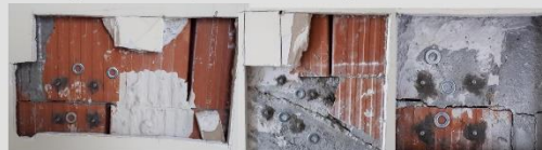
Fig. 3. The location of the measuring network of two methods next to the resulting cracks
