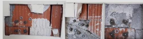
Fig. 3. The location of the measuring network of two methods next to the resulting cracks
